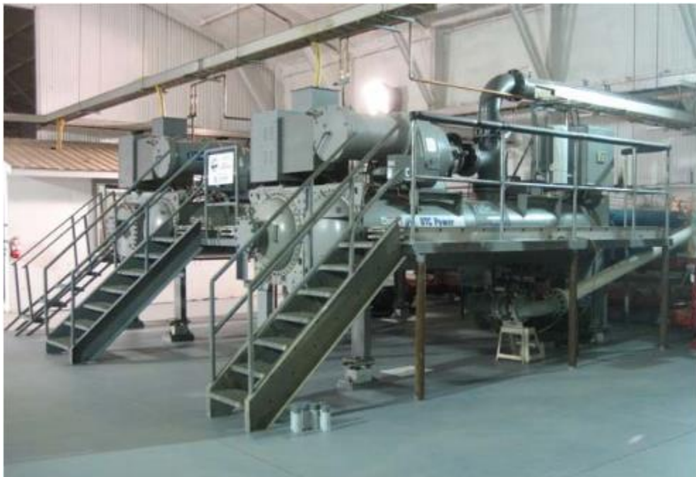
Figure 3 Two 225kW ORC Units at Chena Hot Springs, AK; Electricity from 73 degC warm water (from Holdmann, 2006)
